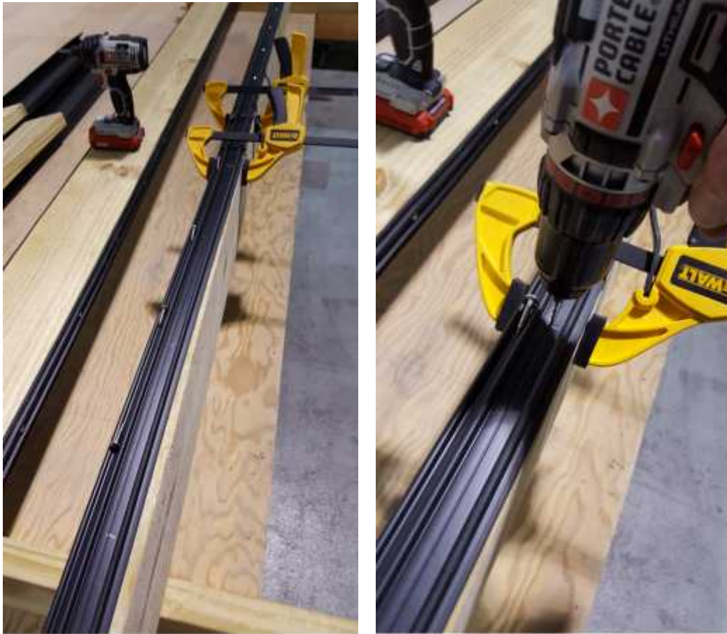
FIG 4 Screw placements are marked and screws are installed. Right, you can see a Drill being used to Pre-Drill a location for a screw. Use a smaller drill bit to allow the screws to grip properly when installed.
