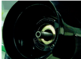
Aft drive adapter incorrectly installed. The propeller will fall off the propeller shaft if run with this incorrect installation.
