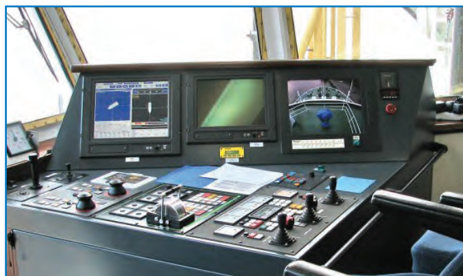
Integrated Power System provides primary and back-up power to critical navigation and safety systems.
