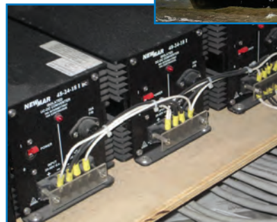
Isolated converters in parallel/redundant configuration deliver noise-free and regulated voltage to propulsion system controllers.
