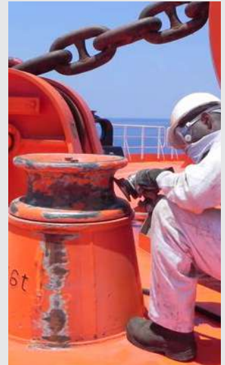
The adhesion and longevity of any paint coating is dependent upon the surface preparation prior to coating.
