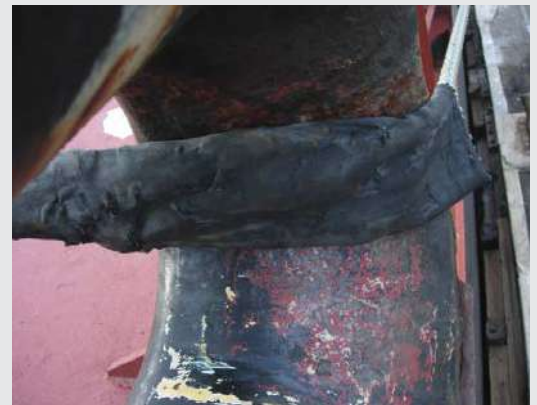
Rough finish as coating wears away.
