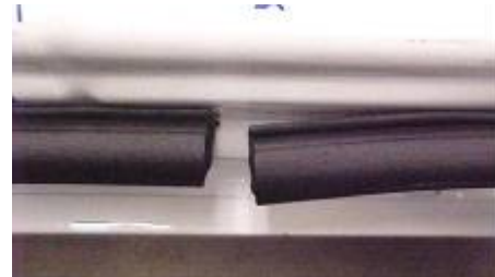
Seal end on the right has crept back and lifted away from painted surface.
