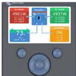
Color Control GX, showing a PV application
